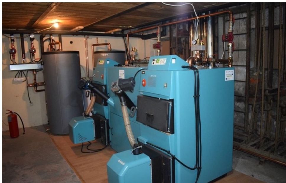
The new boilers powered by wood pellets
