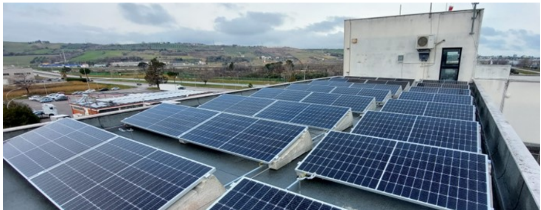
The installed PV plant
