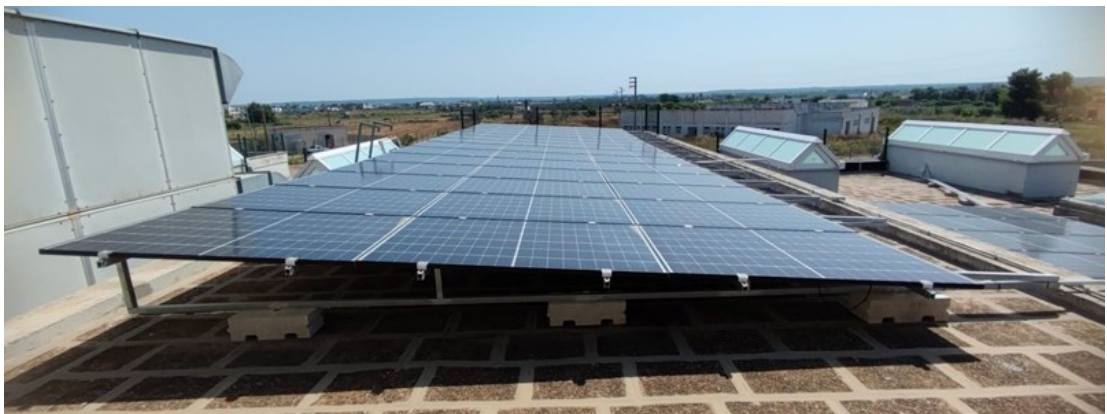
The installed PV plant
